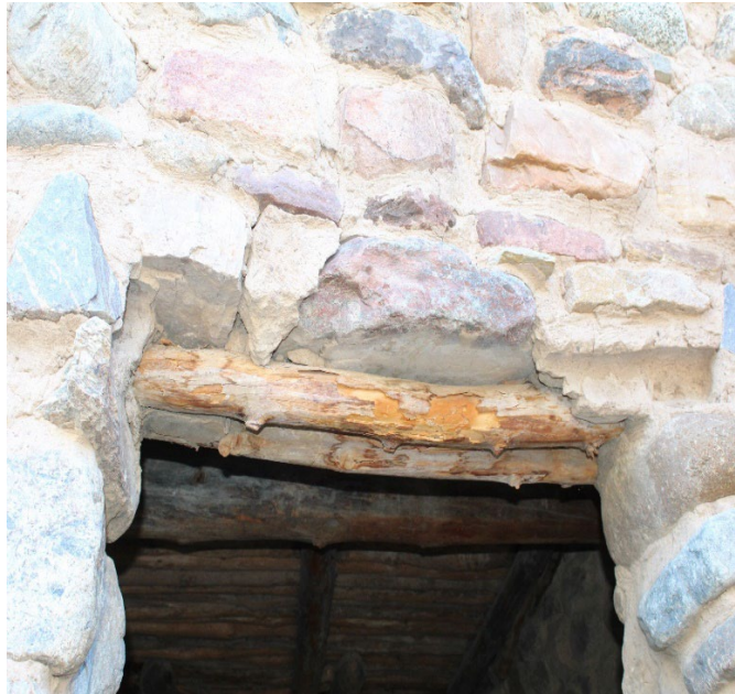
South Building lintel failure
