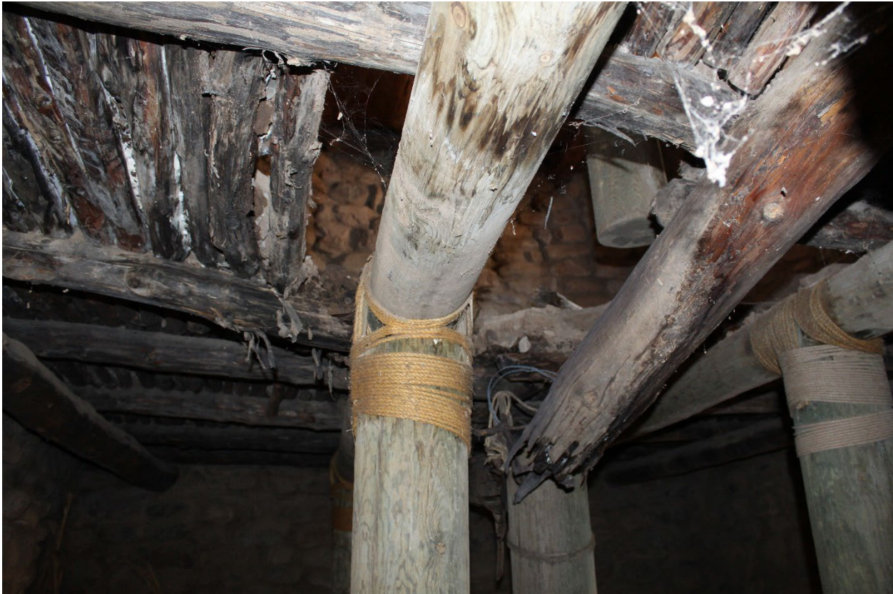
Detail of damaged floor area
